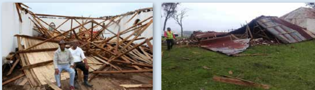
Figure 4: Evidence of wind damage in the Mthatha area of the Eastern Cape Province on 7 April 2018 (Garth Sampson, Port Elizabeth Weather Office)
